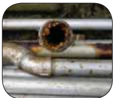
Corroded steel pipe
